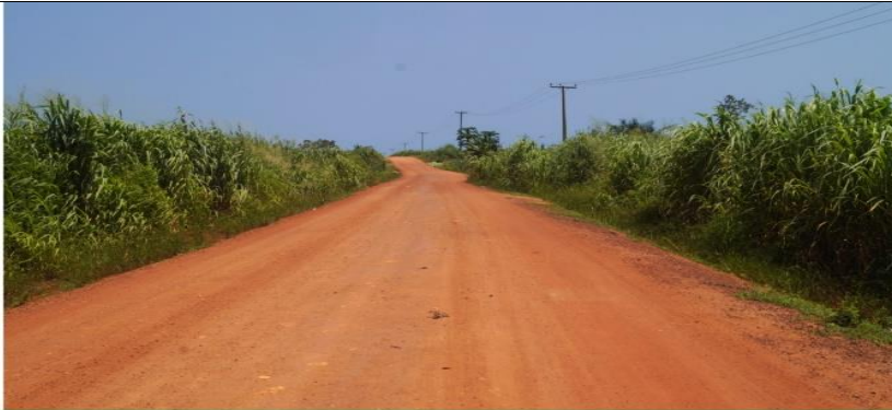
Reshaping of Aburansa to Kafodzidzi feeder Roads (4.1km) and Filing of Culvert
