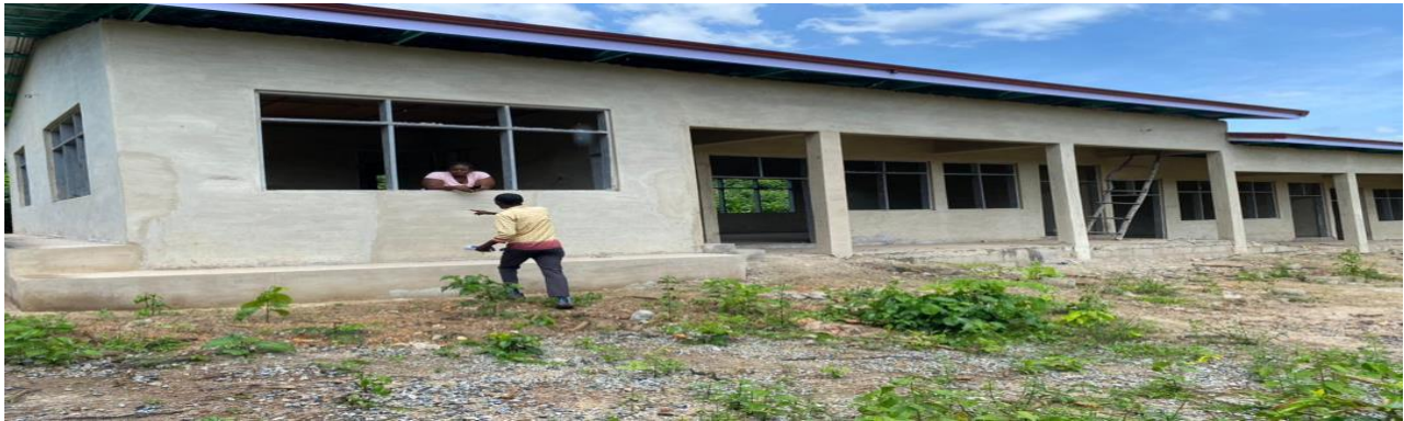
Figure 4: 1No. 3-Unit Classroom Block with 150 No. Dual Desk, Office Tables and Chairs at Essiam (On-going)
