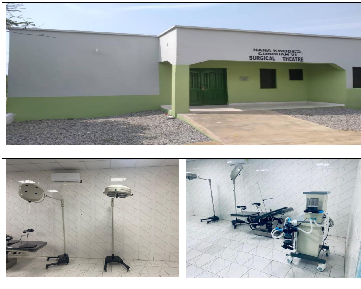
Figure 1:1 Completion of 1No Operating Theatre with 1No Theatre Table, 2No Theatre Lights and 1No Anaesthesia Machine at Elmina Polyclinic
